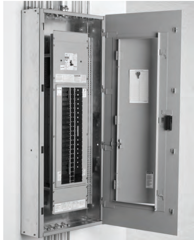
Trim Hanging on Surface Mounted Box
