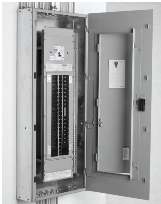
Trim Hanging on Surface Mounted Box
