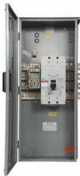
Main Circuit Breaker
