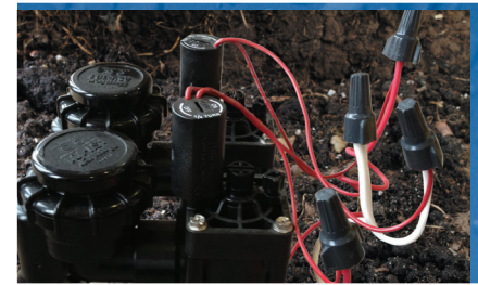
irrigation and sprinkler systems
