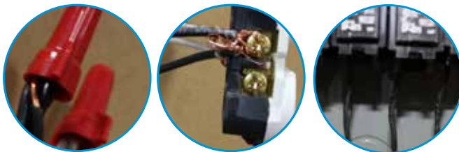
Improper solid wire connection.
